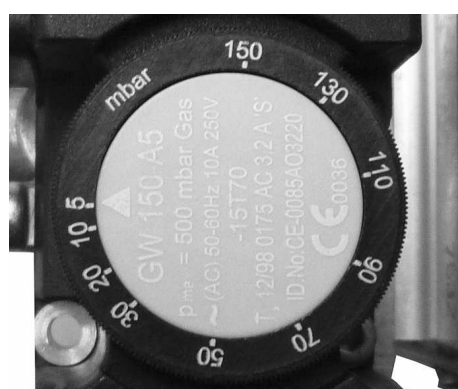
Setting the gas pressure monitor to Minimum (5 mbar at MBC65 1/2")
